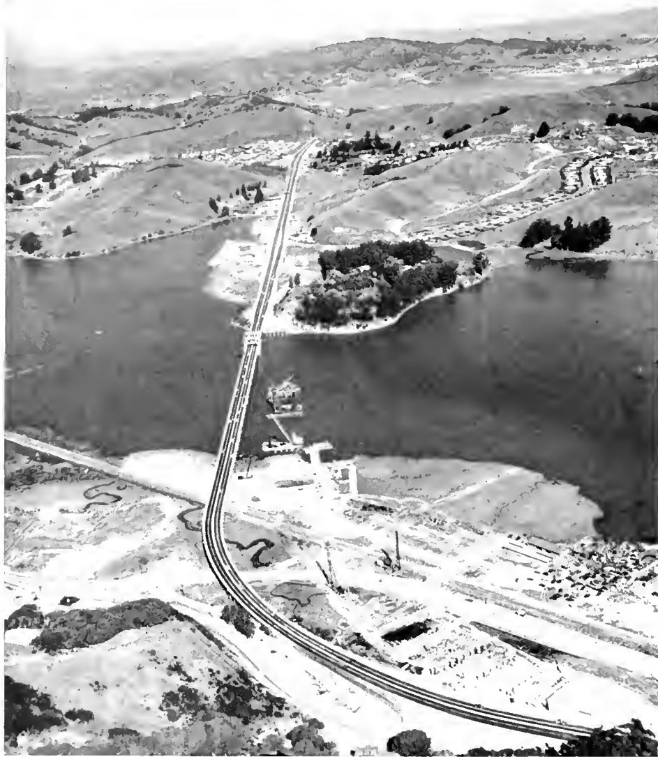
Construction operations on foundations for new bridge across Richardson Bay in Marin County. When the new six-lane divided facility is completed the existing timber bridge which has reached the end of its useful life will be removed.
